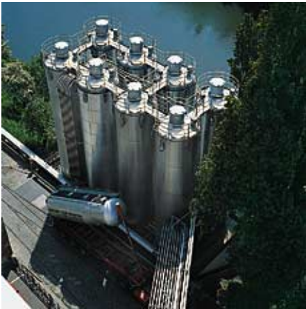
Outdoor silos of nickel chromium steel, partly insulated.
